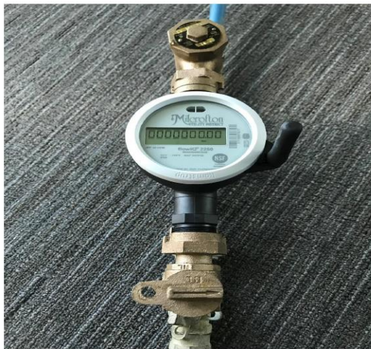
Advanced Water Meter Infrastructure water meter in the new meter setters and piping.
